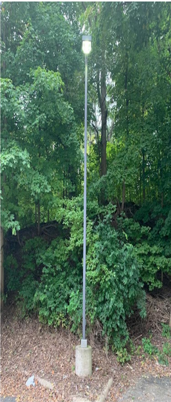
Lights (7) -Parking Lot
