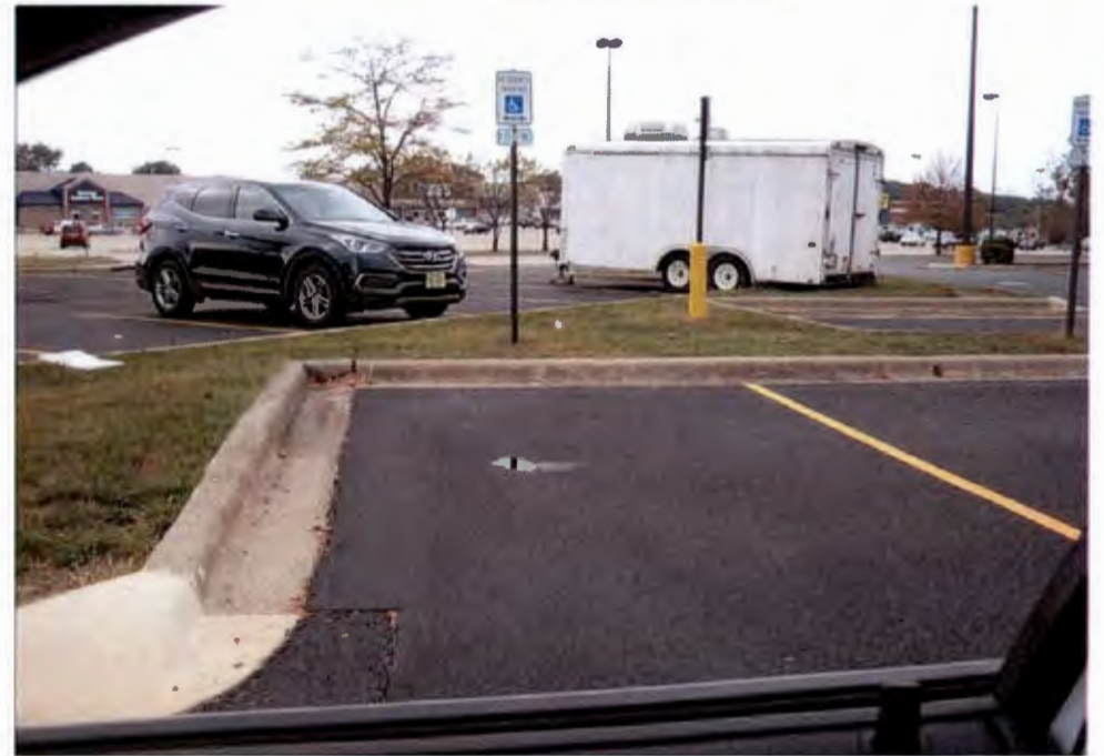
Disabled Space improperly striped (no access aisle) - Five Below
