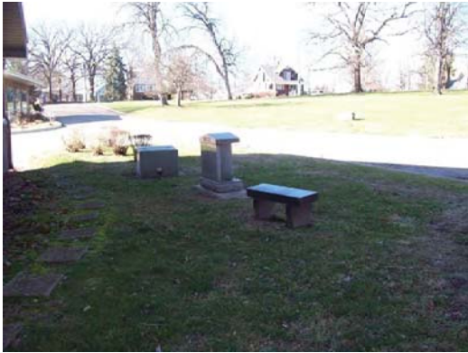
STANDING NORTHEAST OF THE SITE AT THE EXISTING ELECTRIC TRANSFORMER (LOOKING WEST)
