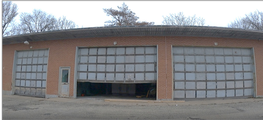
Figure 14. Building 8-9 on the Keller Station Site presented vacant and deteriorated conditions (photo: 12/7/2021).
