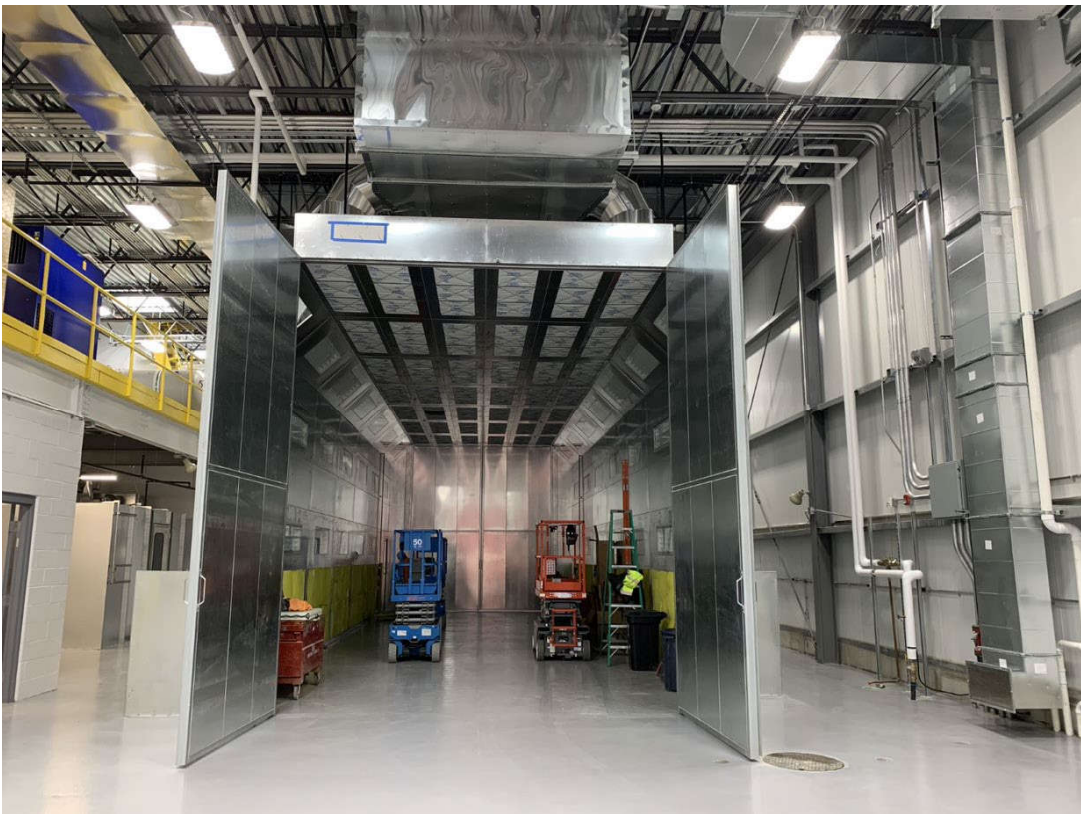
Picture of the new paint booth in the new body shop from Phase A construction.
