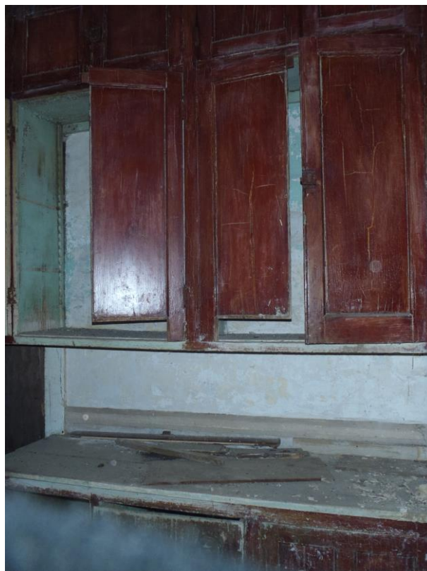
Condition of remaining kitchen cabinets indicating needed replacement
