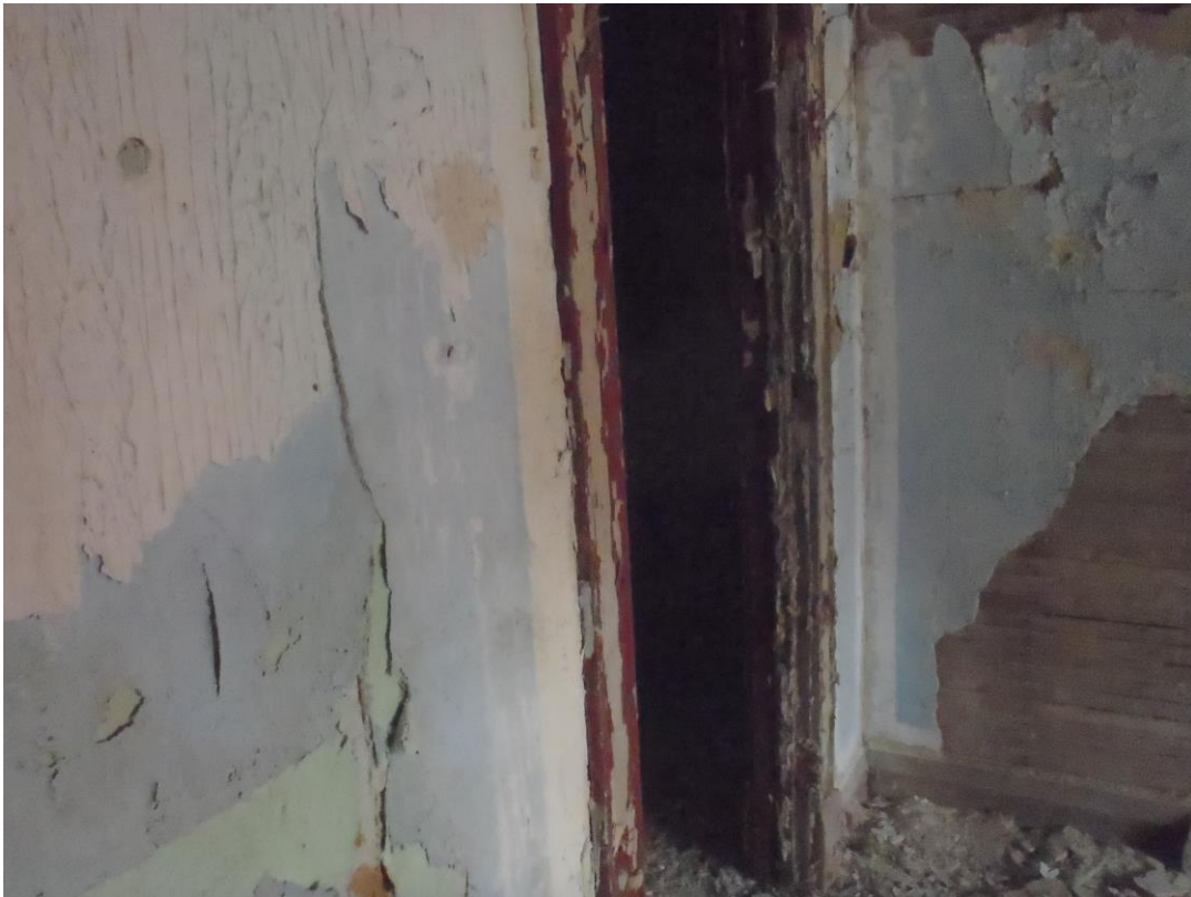
Peeling paint indicating the need to replace wood work and plaster (scaling paint on wood work is generally an indicator of lead based paints)
