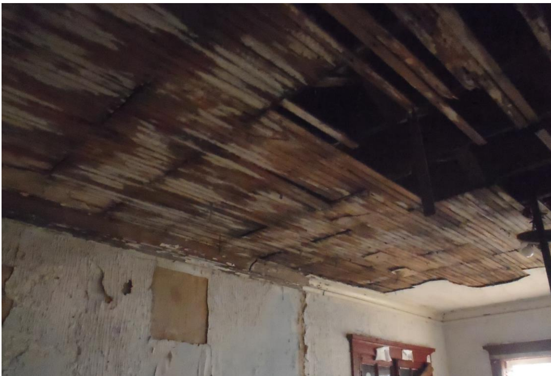
Deterioration of ceilings showing need to add gypsum board
