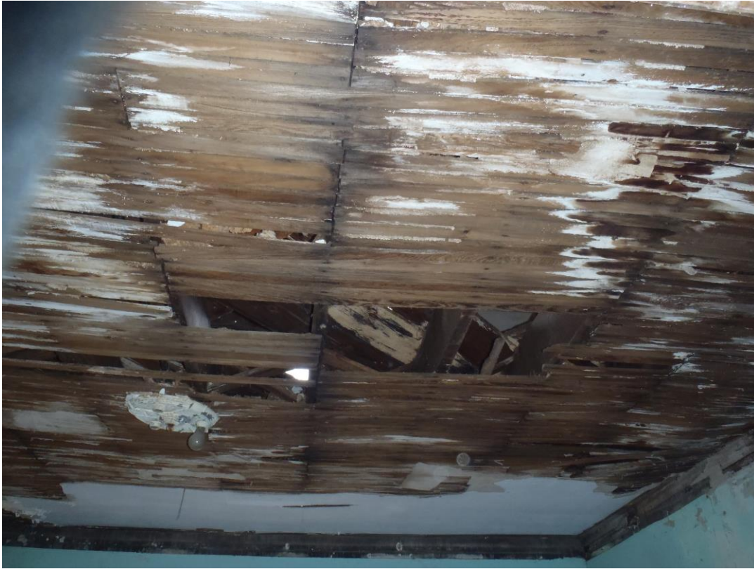
Deterioration of ceilings showing need to remove lath boards and replace with gypsum board
