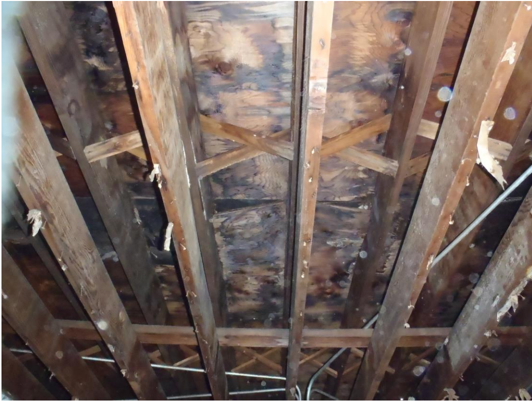
Water damaged and deteriorating roof sheathing indicating the need to replace the roof sheathing
