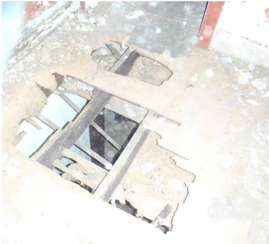
Hole in floor shows the need for repair and/or replacement of some floor framing members.
