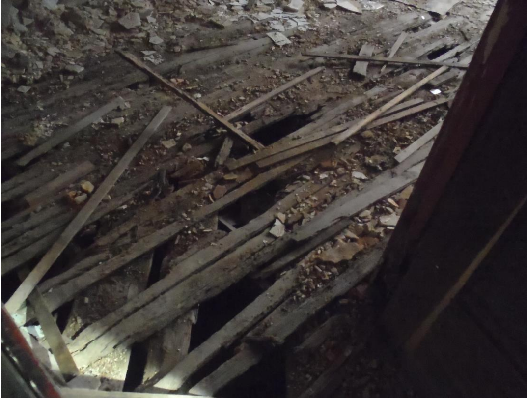
Existing deteriorated flooring needs to be removed and replaced.
