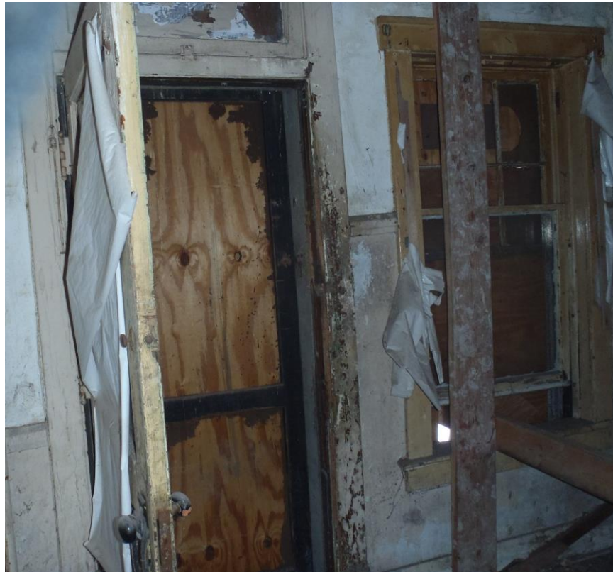
Interior view of door and window showing damaged hardware that will require replacement and peeling paint on the wood that will require replacement of the wood trim and abatement on the window sashes
