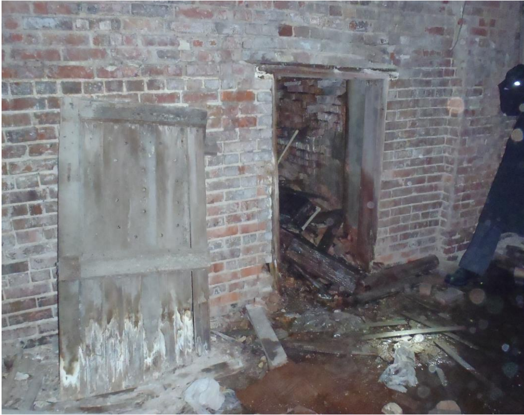
Water in basement (Infiltrating from near damaged exterior wall)
