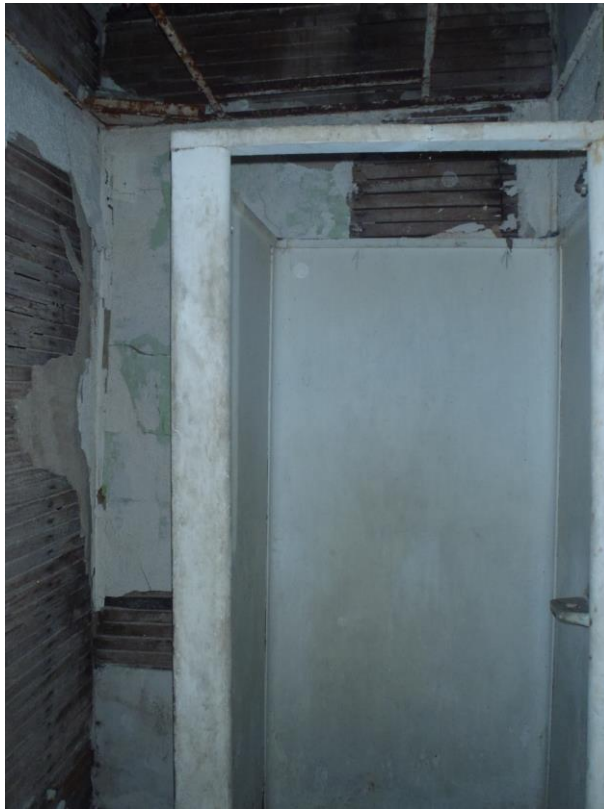
Remaining shower needing replacement
