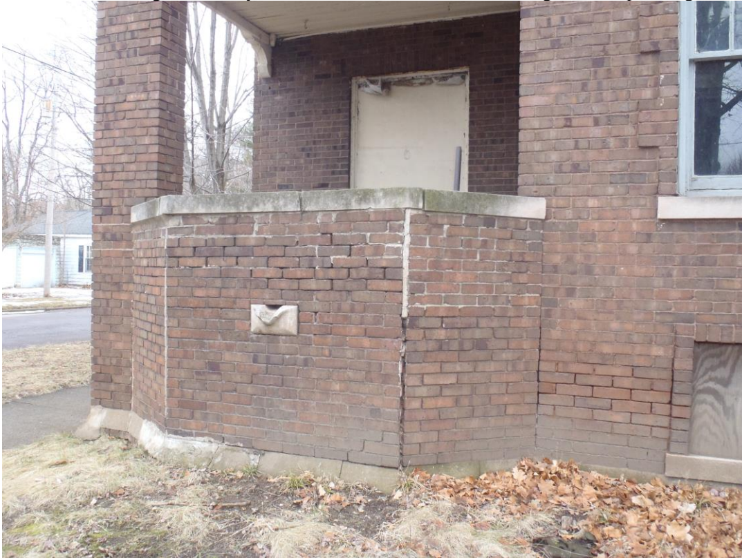
Exterior balcony needs masonry repair and tuckpointing
