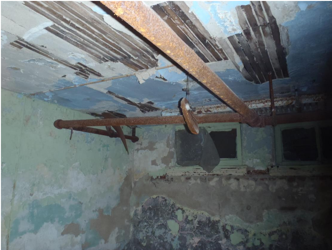
Heat piping is rusted and in need of replacement
