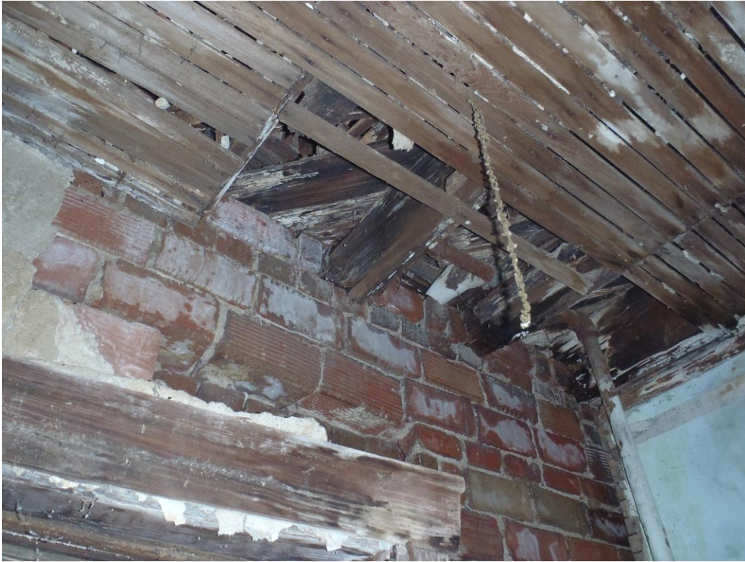
Water damaged flooring and joists indicating the need for replacement of flooring and joists
