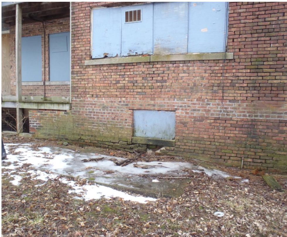
Water damaged masonry (missing brick and mortar)
