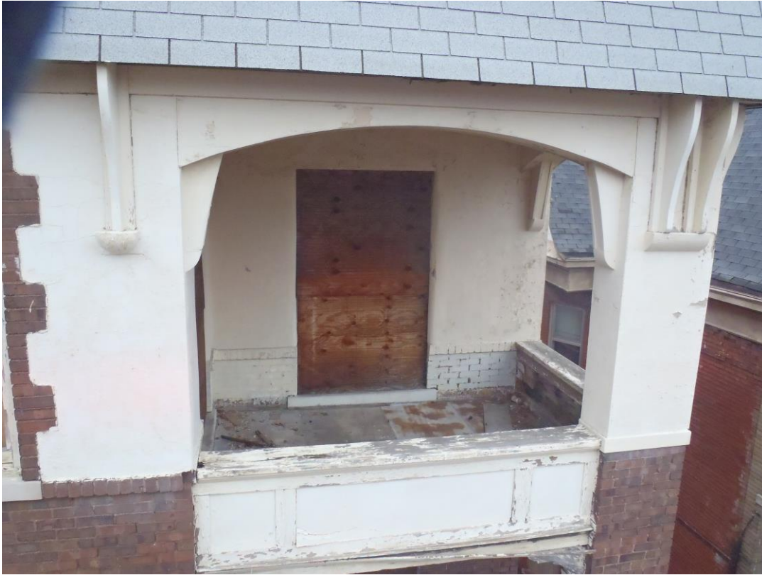
Exterior balcony and exterior wall showing peeling paint and damaged wood trim
