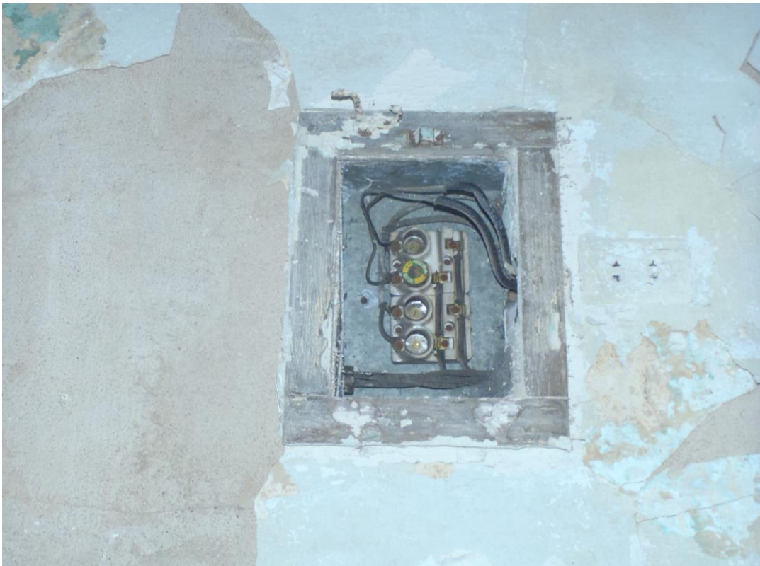
Existing unit fuse box needs to be replaced
