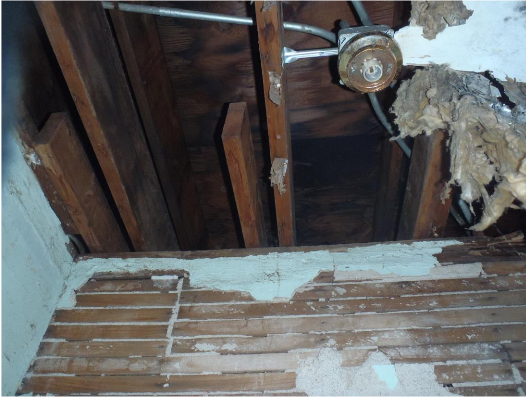
Electrical conduit potentially salvageable, but it is likely wiring will need to be replaced
