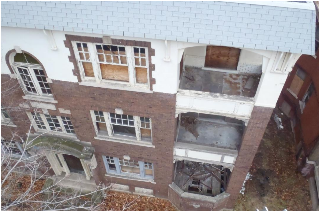
Exterior balconies and windows will require various levels of repair, including framing replacement, window frame and sash repair, glass replacement, and painting.
