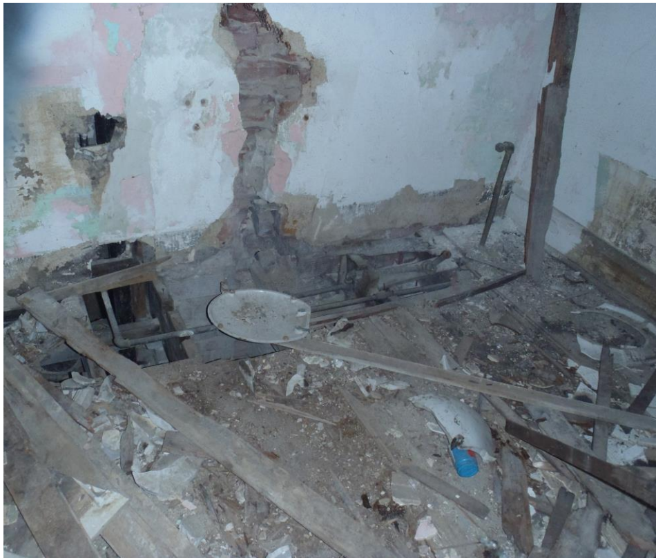
Hole in floor showing need for repair of some floor framing members
