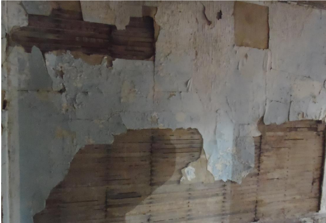
Condition of plaster walls indicating need to replace with drywall
