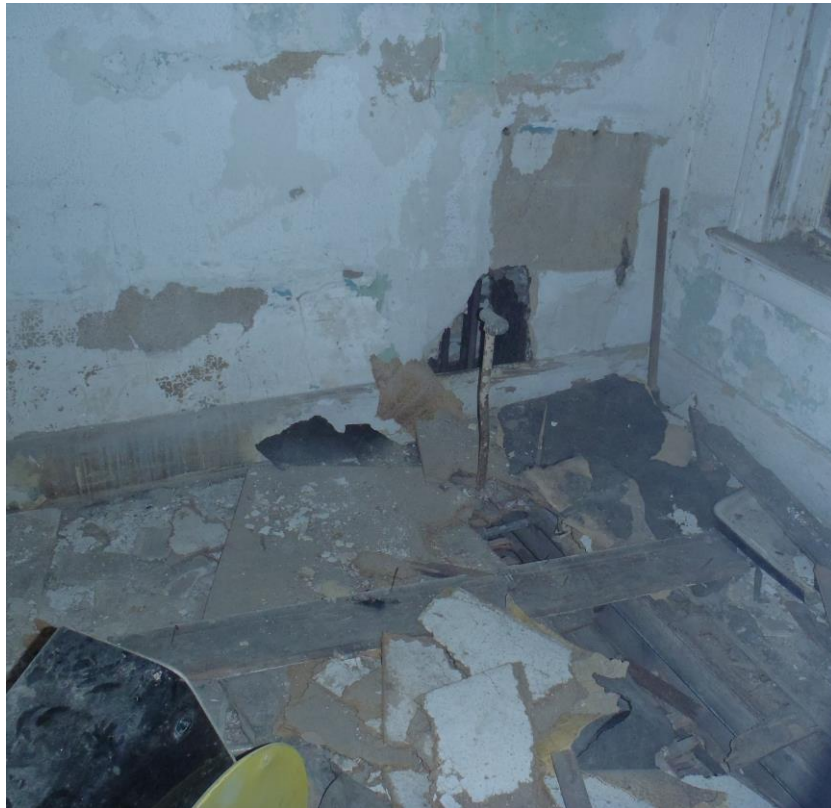
Water piping in poor condition – needs to be replaced
