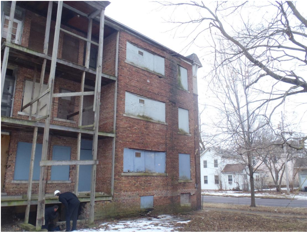
Back wall showing water damaged masonry all the way up between the windows. Also, note missing stairs
