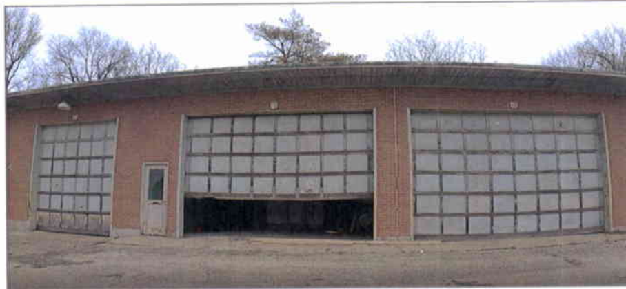
Figure 14. Building 8-9 on the Keller Station Site presented vacant and deteriorated conditions (photo: 12/7/2021).
