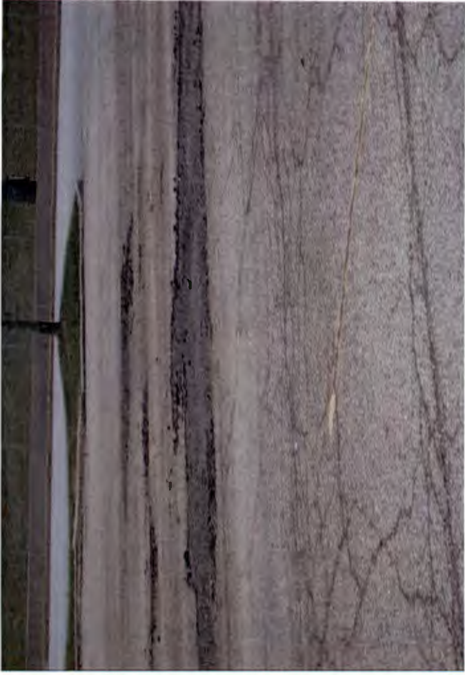
Unmaintained parking surface
