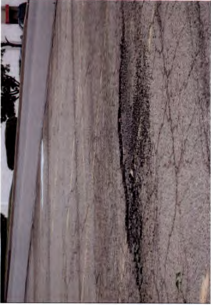
Unmaintained parking surface
