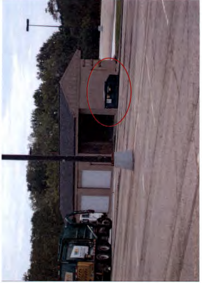
Unscreened dumpster and unmaintained parking surface
