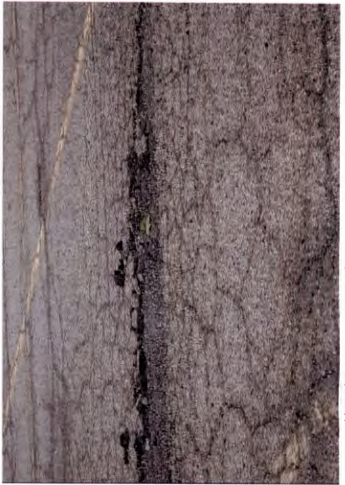
Unmaintained parking surface
