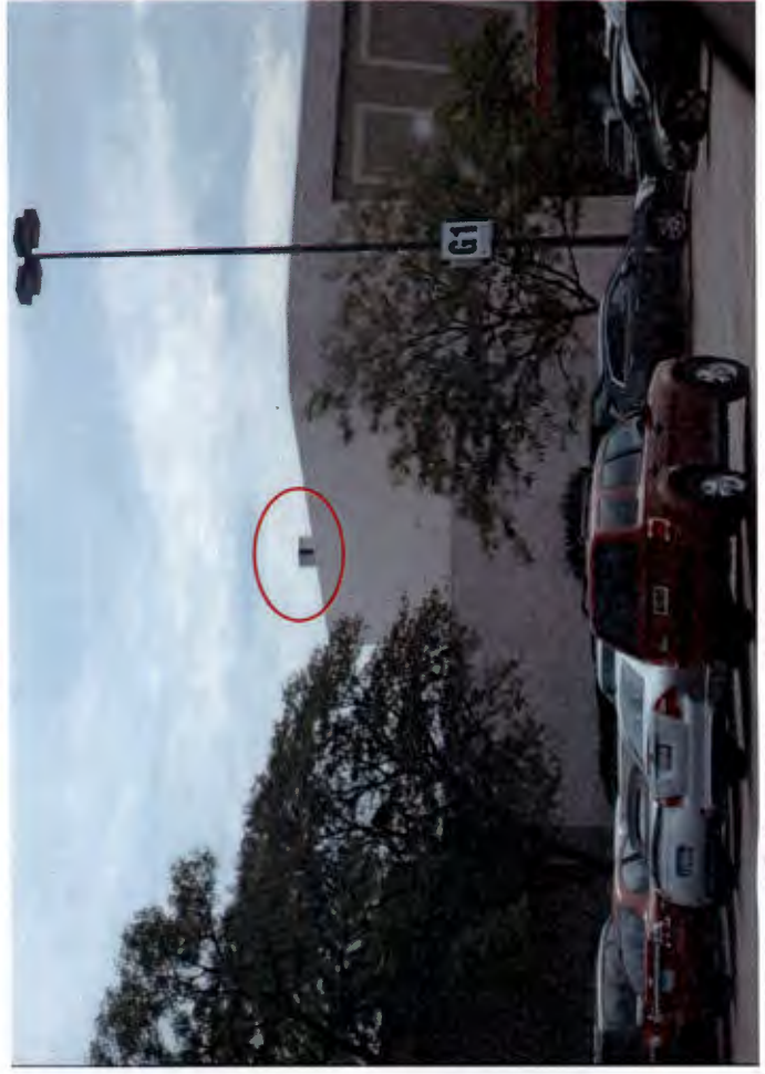
Visible roof-top HVAC Unit
