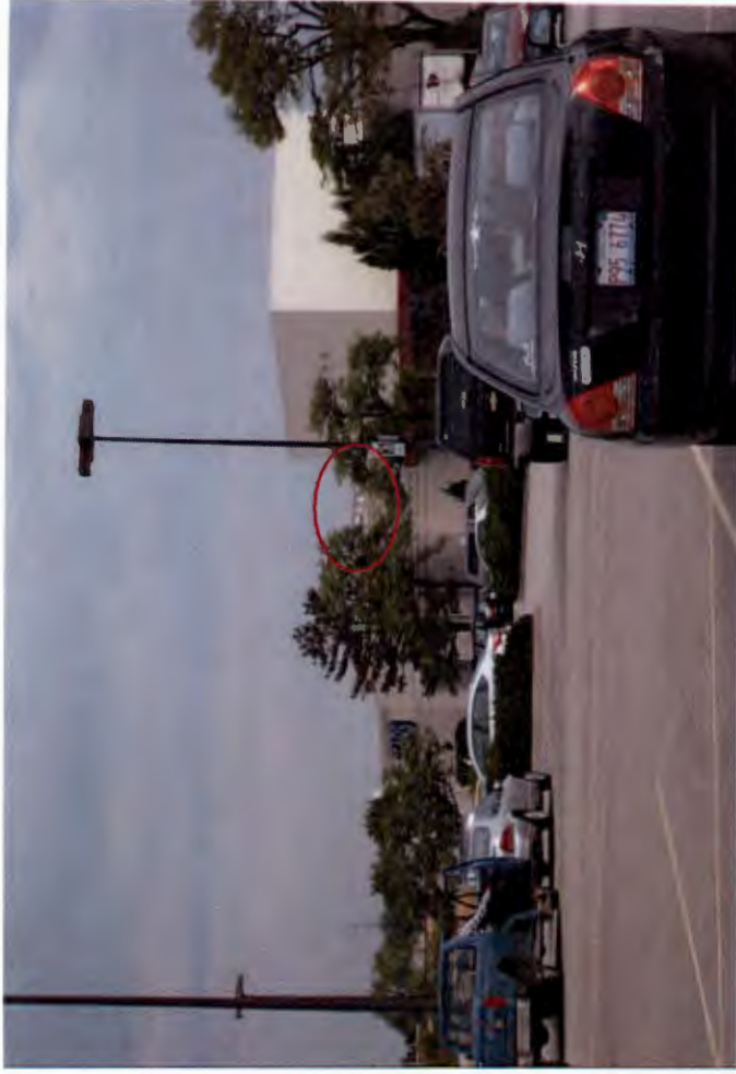
Visible roof-top HVAC Unit
