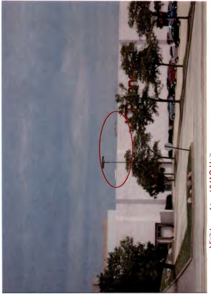
Visible roof-top HVAC Unit
