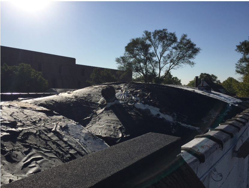
Photo #7 Failed Roof
