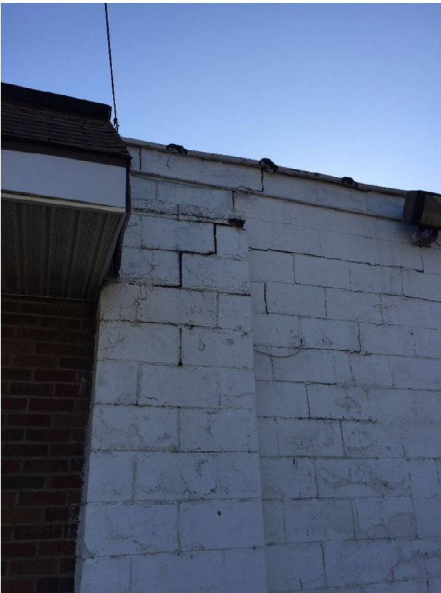
Photo #4 Cracking in 1 st pilaster
