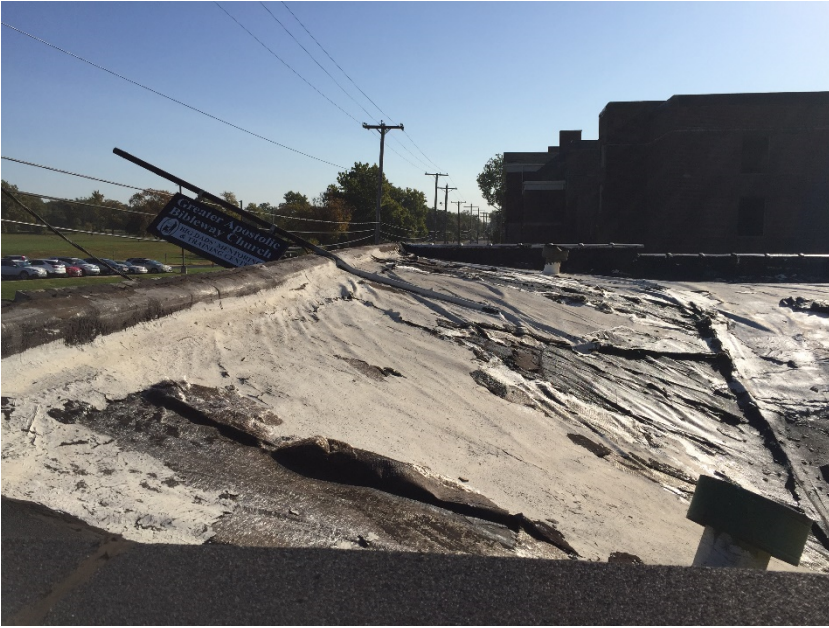
Photo #6 Failed Roof
