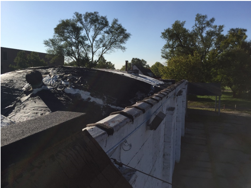
Photo #8 Failed Roof
